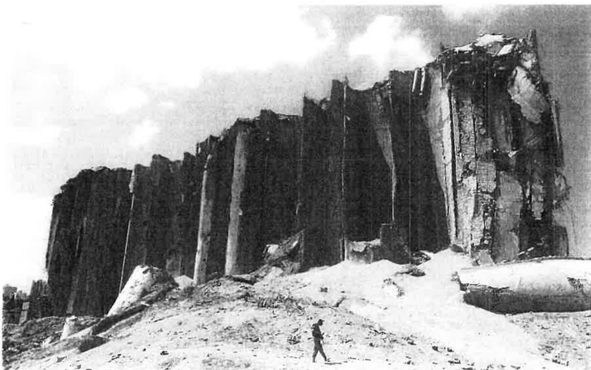
Figure 4. A Front View (Looking to the West) Showing the Damaged Silos
